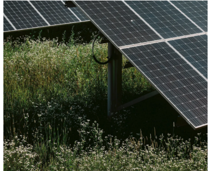
Engie solar panels at the site of the former Mount Tom coal plant in Holyoke, Mass. Simon Simard for The New York Times
